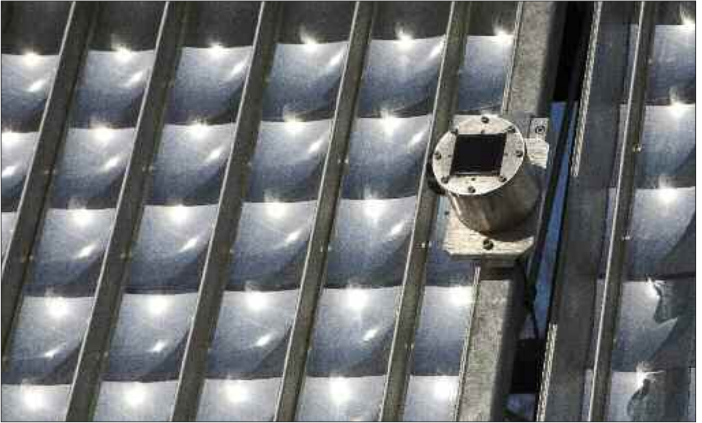
Tracking system with solar camera
